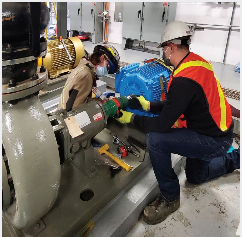
Figure 1. Technicians install and perform an alignment for a new premium efficiency motor, selected for energy savings on a pumping application. Courtesy of Motion Repair & Services
